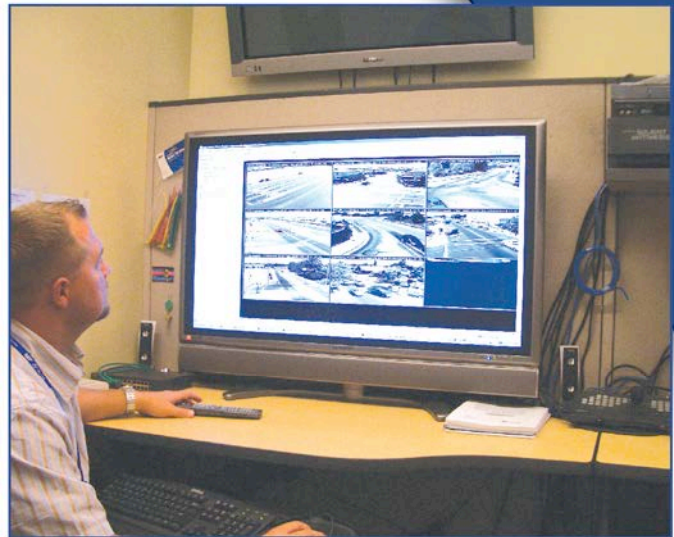
MPEG-4 cameras provide a clear, smooth, real-time video of each intersection, allowing engineers to make intersection adjustments.
